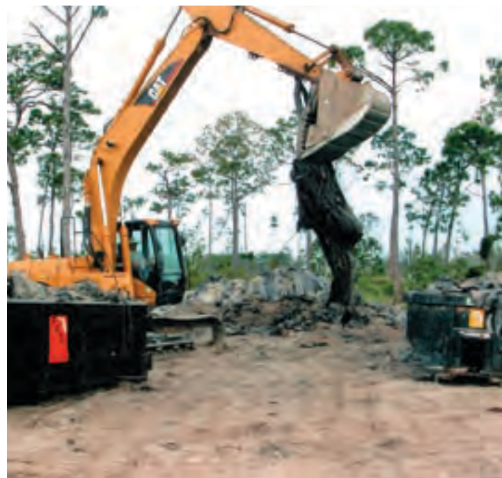
The removal of temporary roads constructed from tire mats is the last remaining heavy equipment operation.
